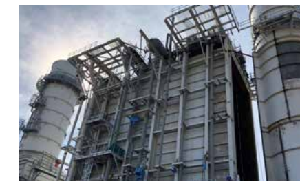
Closure of the Ensenada Barragán Cycle (280 MW).
