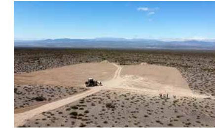
Zonda Solar Farm (100 MW).
