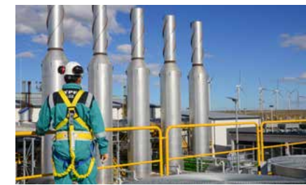
Manantiales Behr Thermal Power Plant, 58 MW.
